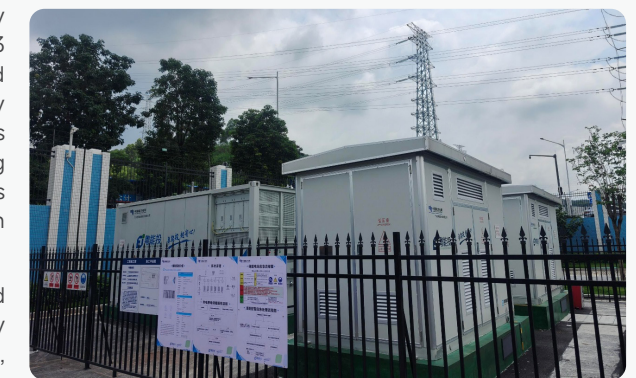
Energy storage power station
